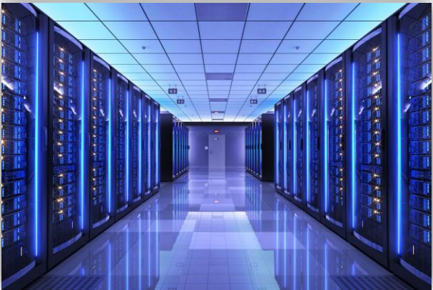
Data Center Cooling
